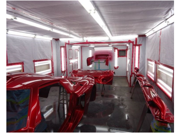
Spray paint booth
